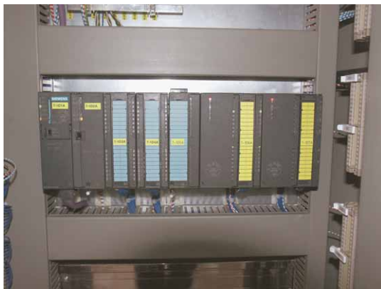
Figure 4: Fail-safe PLC S7-300 of RSSM.
