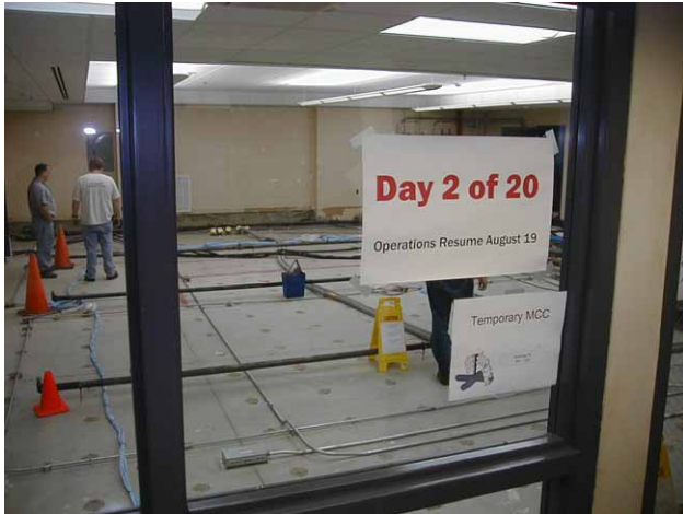
Figure 2: All remaining equipment removed in first 2 days. One can also see the 1 st phase ceiling effort.
